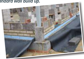
Thermal imaging: This show heat lost through the bottom of a standard wall build up.
